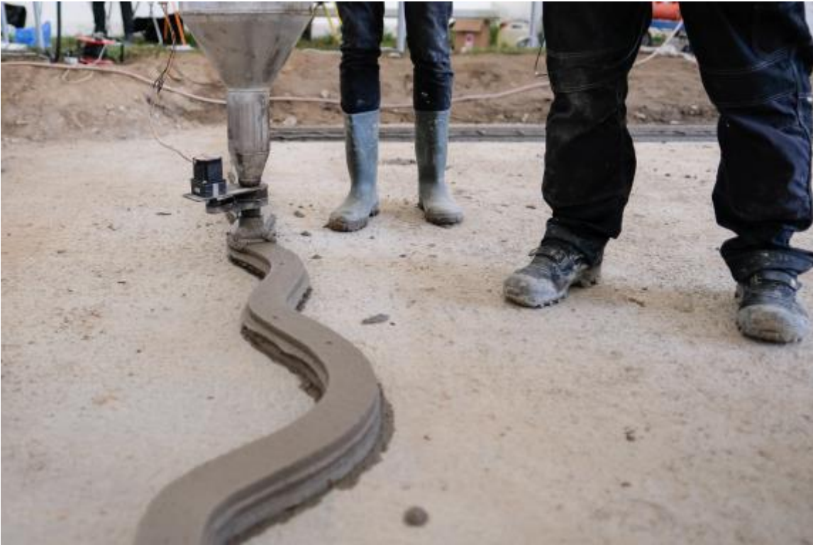
Start of the 3D printing of the upper part of the foundation of The BOD – Europe's first 3D printed building
