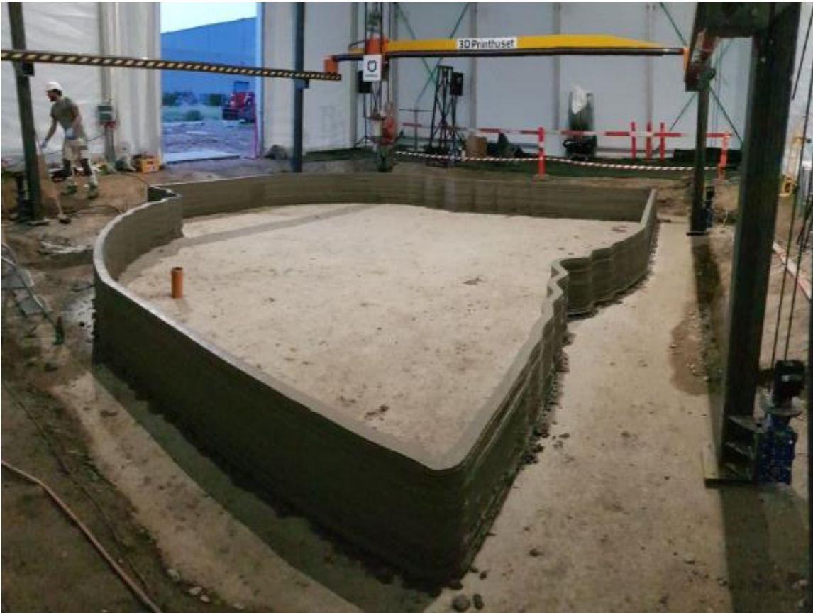
3D printing of the upper part of the foundation of The BOD was finished later the same day.
